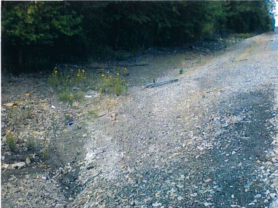
Date: 4/21/2010 Time: 2:45-4:00 PM Direction: Northwest Photo by: M. Stevenson Exposure #: 009 Comments: View from Sesser side of RR tracks. Culvert is located in bottom left of picture. Some scattered debris among the broken branches and vegetation.
